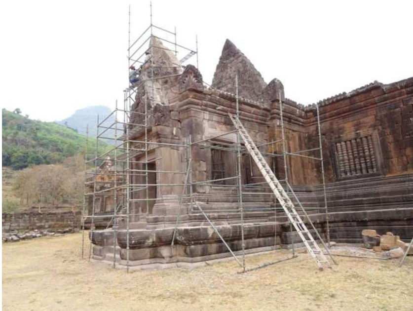
15. Restoration of the North Quadrangle by the India-Laos Cooperation Project is now largely completed (source: W. Logan).
