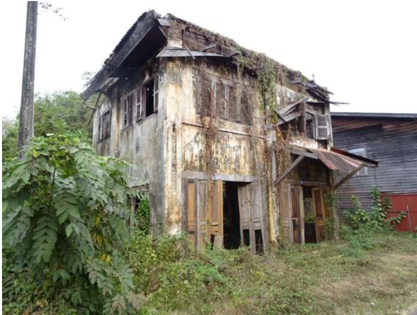
11. One of Champasak town's last remaining colonial-style buildings in derelict condition (source: W. Logan).
