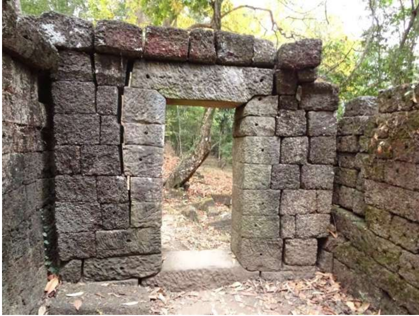
17. Tomo Temple, on the east side of the Mekong, has yet to receive major funding for restoration (source: W. Logan)
